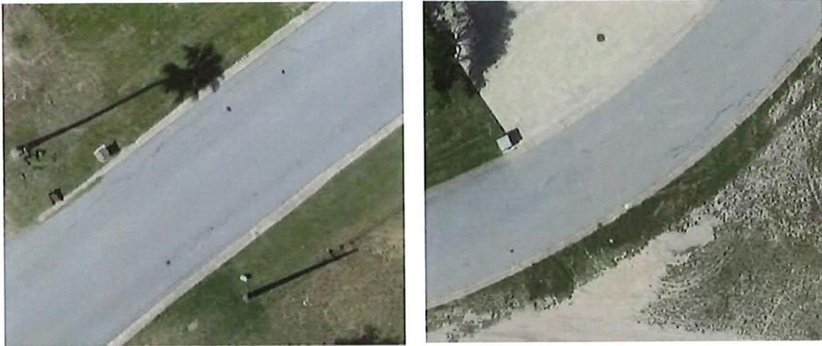
Figures 3 & 4. Examples of streets classified as being in "Good" condition. Here there is evidence of minor cracking. However, the cracking can be addressed with minor seal coating.
