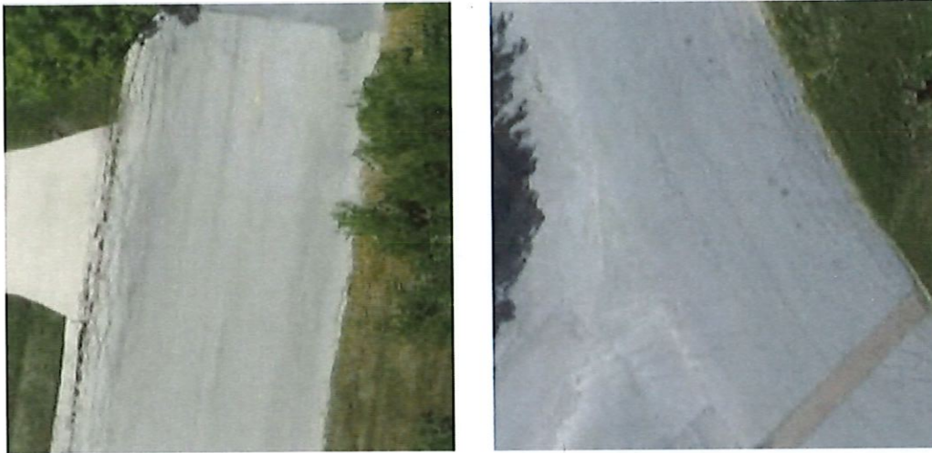
Figures 5 & 6. Examples of streets classified as being in “Fair” condition. Here there is a moderate level of cracking or deterioration throughout the whole street, however the thickness of the cracks is still relatively low.
